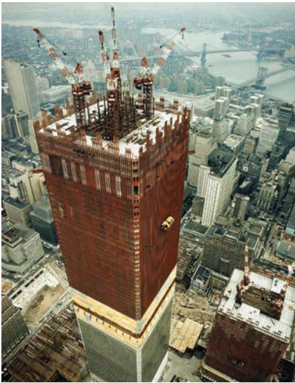
The World Trade Center under construction in New York City in the 1970s.
