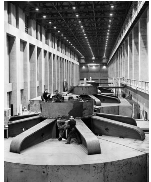
Hydroelectric generators at the Grand Coulee Dam.
